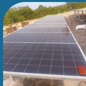
DOMESTIC ROOF TOP SOLAR
